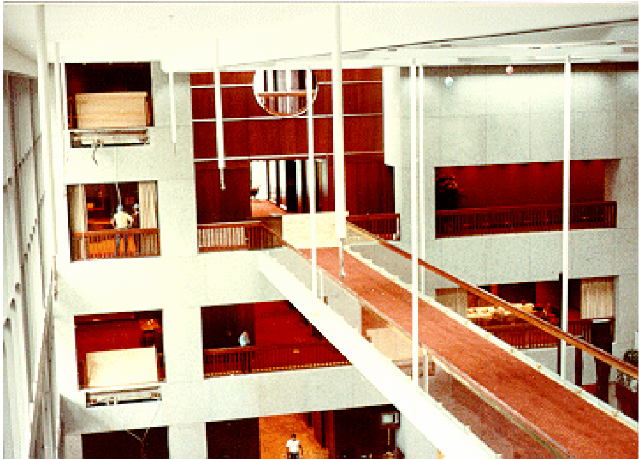
Figure 10 Surviving 3 rd Floor Walkway
